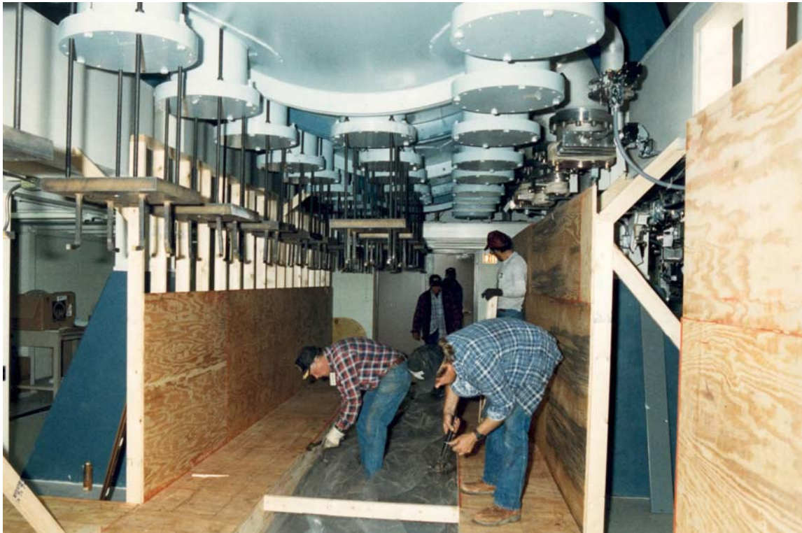
Forming the mass below the existing vacuum chamber. The vacuum chamber itself is supported by columns on the facility floor.
