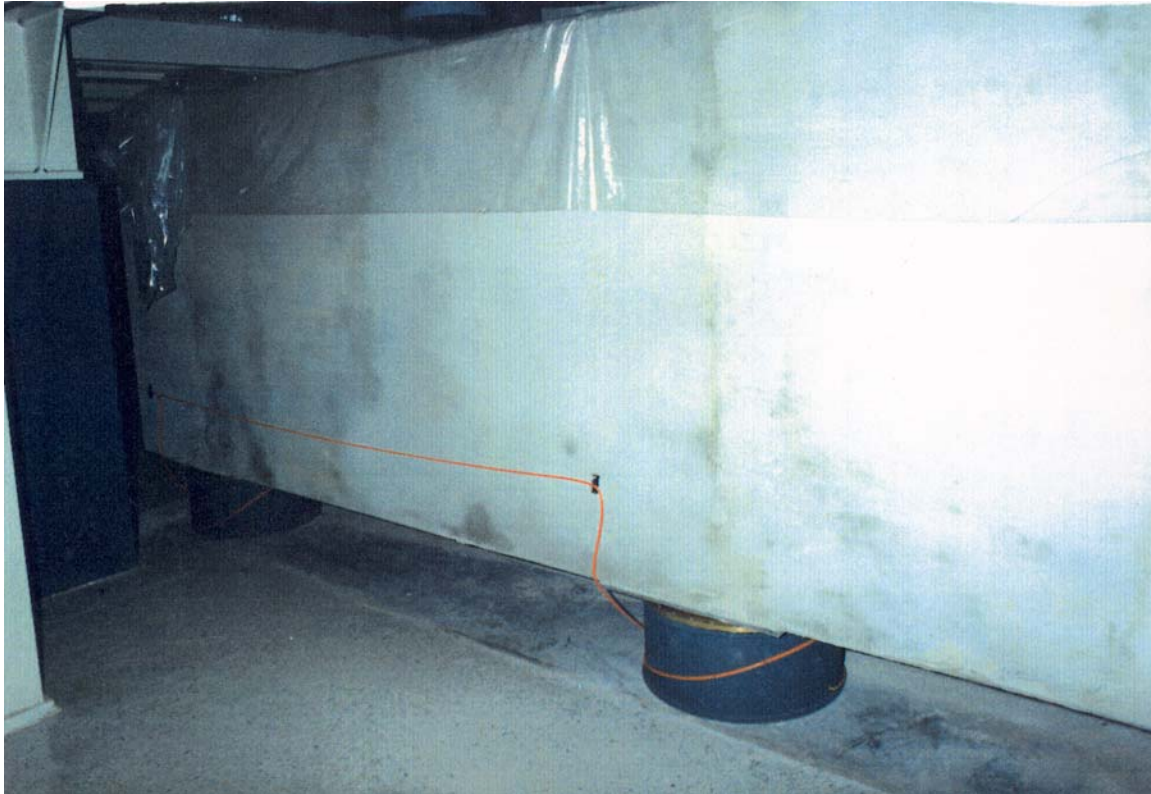
Completed seismic mass supported by pneumatic isolators.
