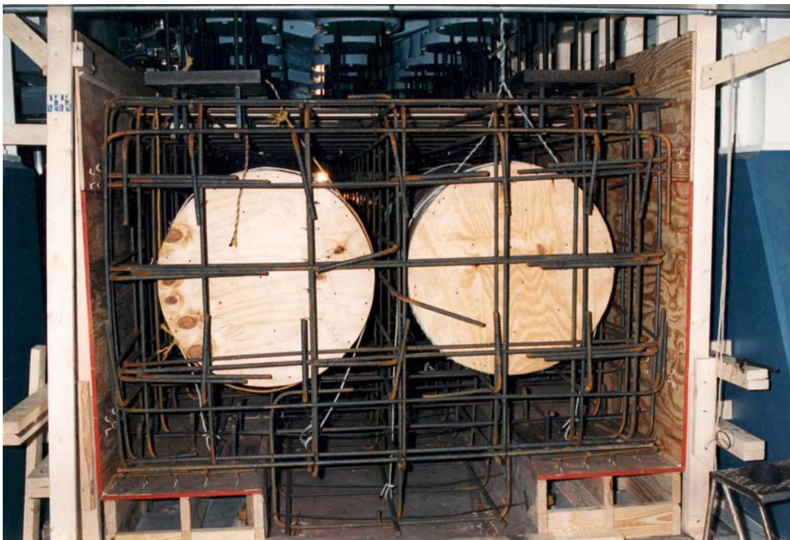
End view of the mass being formed. Note the hollow tubes positioned at the neutral axis of mass. The tubes reduce the overall weight to be supported and increase the stiffness (dynamic response modes) of the mass.
