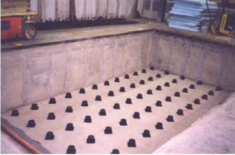
Foundation isolated on INFAB™ elastomeric isolators.
