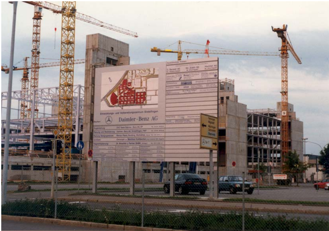
Construction site of the new Mercedes-Benz research and development facility in Sindelfingen, (Stuttgart) Germany. At one point, the second largest construction project in Europe.
